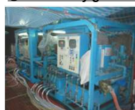
Automatic chemical mixer
