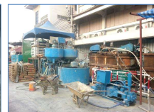
Plant facilities for drilling
