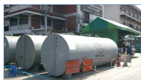
Tank for water glass (sodium silicate)
