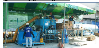
Plant facilities for primary injection
